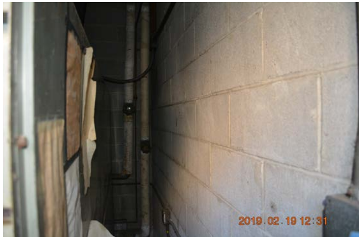
Photo 20: Air handler room limited access around equipment. Replacement would require partial removal of the exterior wall.
