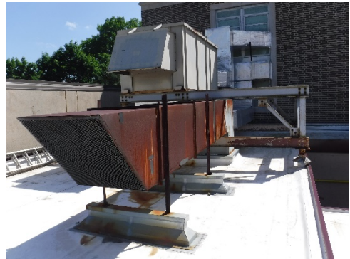
Outside Air Duct
