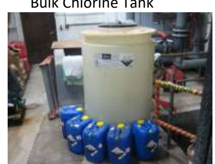
Bulk Chlorine Tank
