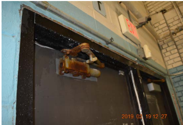
Photo 22: Pair of exit doors toward Elliott Place. Door hardware base metal suffers in the corrosive atmosphere. In cool weather, the refrigerated metal surfaces have water freely condensing on all surfaces.
