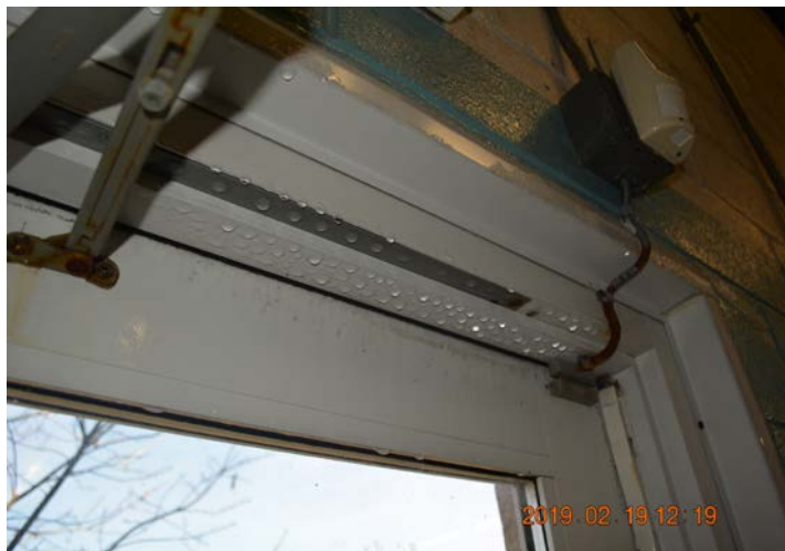
Photo 23: Exit door toward field. Condensed moisture is readily visible. Any carbon steel base metal items quickly corrode under this aggressive condition.
