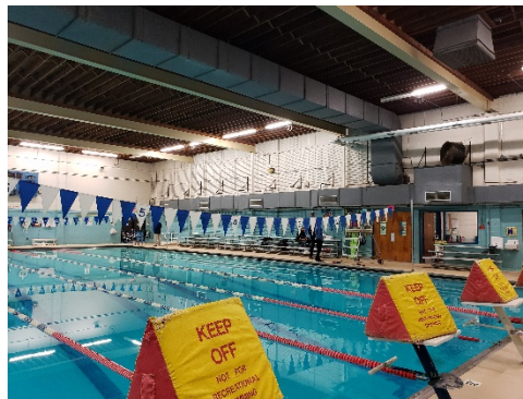
Return Air Duct and Exhaust Inlet
