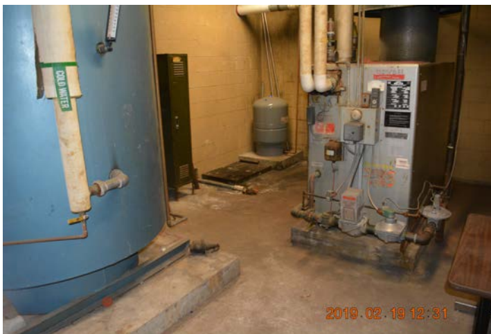
Photo 18: Boiler Room. This unit supplies heat for pool water, pool space room air heating, and it also supplies domestic hot water to the Elliott wing of the High School.
