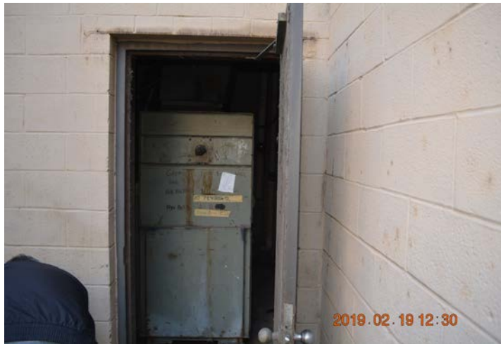
Photo 19: The existing air handler machine room is only accessible from the exterior door shown here. Minimal space is available around the equipment, barely sufficient to squeeze along one side and one end. Serviceability is impaired.
