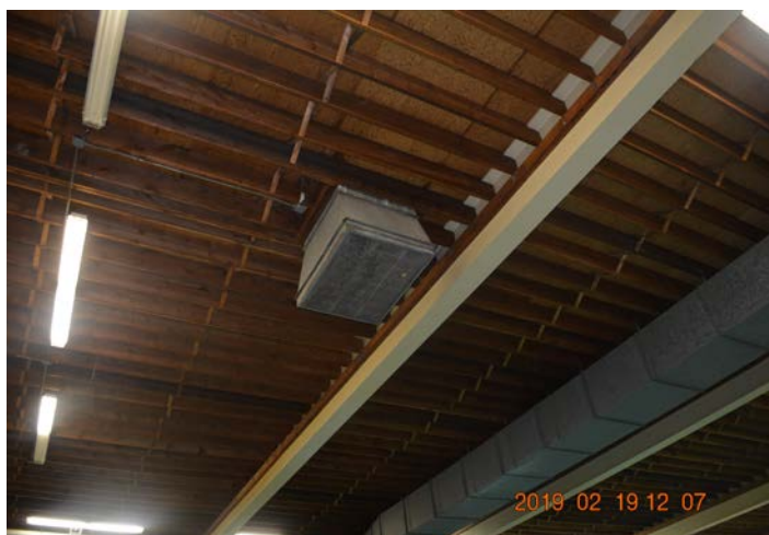
Photo 12: Single point exhaust register at roof. This system pulls out room air with its odors and heat. The existing exhaust setup has no means for recovering the thermal energy in the air being pulled out and exhausted to the exterior.
