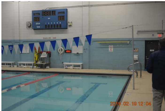
Photo 11: Opposite End wall, with Scoreboard: Note the pole supporting the cross pool flag line cable. The guy cable extending from pole top to the right side is actually fastened to the wall mounted duct work that is just outside the photo edge. It really should be routed properly to a wall anchor point, like that on the other side.
