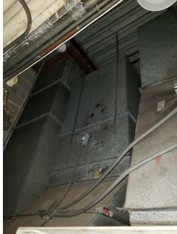
Outside Air and Return Ducts
