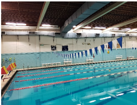
Supply Air Duct
