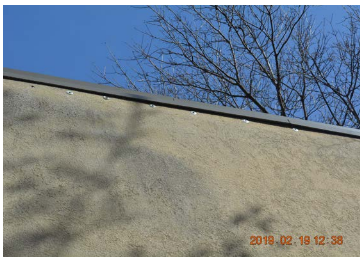
Photo 3: The top edge of three wall shown in Photo 1 has been mechanically fastened over the delaminated zone to prevent gross separation until the wall system can be replaced.
