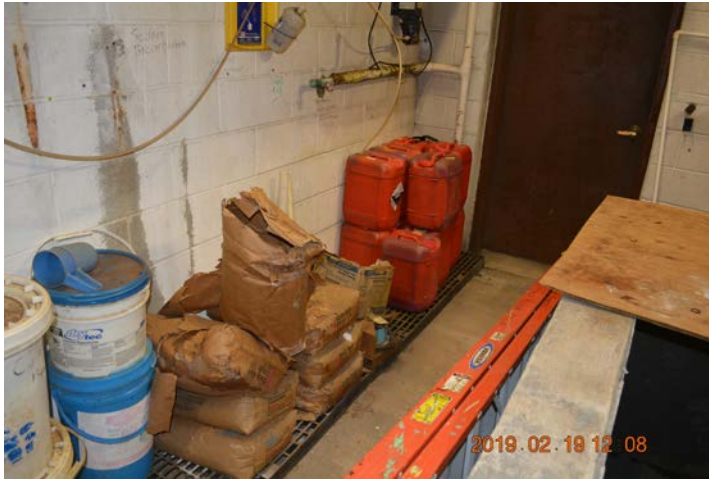
Photo 16: Exposed chemical storage area in the filter room.
