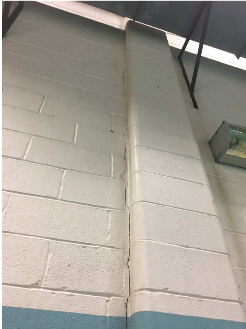
Photo 1 – Crack between pilaster and masonry. Typical at pilasters on exterior side of pool enclosure
