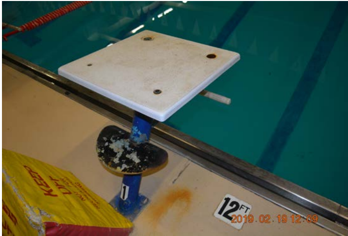
Photo 13: Typical starter platform. These are of rigid permanent type, non-removable. Finish on bases are in poor condition. Hardware is corroded. Foam safety cps are in poor condition also.
