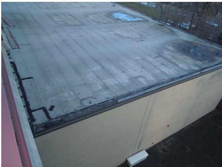
Photo 9: Western section of the main pool roof as it is today. Dark seam repairs are visible in lower left corner, and ponding is observed at the southern edge. The lighter shading strips running perpendicular to the roll lap lines are the high points above the steel girders below. Those lines of less deflection in the roof deck make the ponds occur in localized depressions between the main girder lines. A new roof application could utilize tapered insulation along with local sump kits at the drains to eliminate the ponding.
