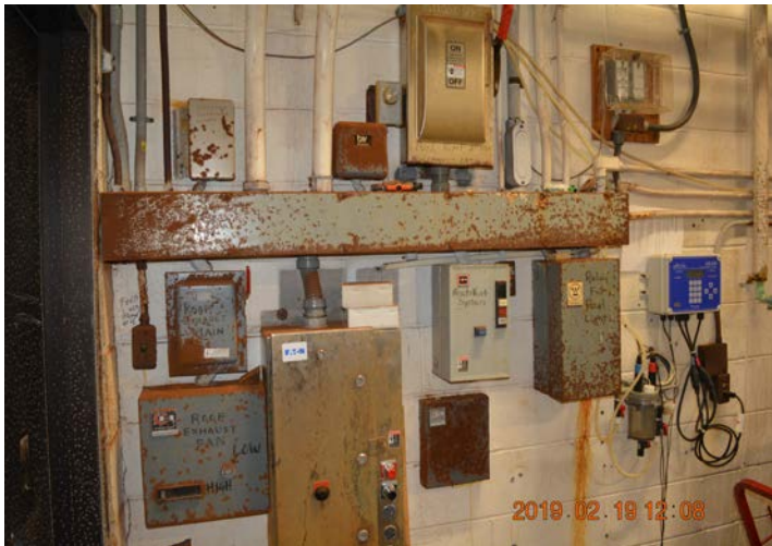
Photo 17: Electrical Center within the Filter Room, immediately adjacent to the chemical storage location. Metal components are incurring extreme corrosion. Replacement of selected devices has become necessary in the past in order to restore functionality.
