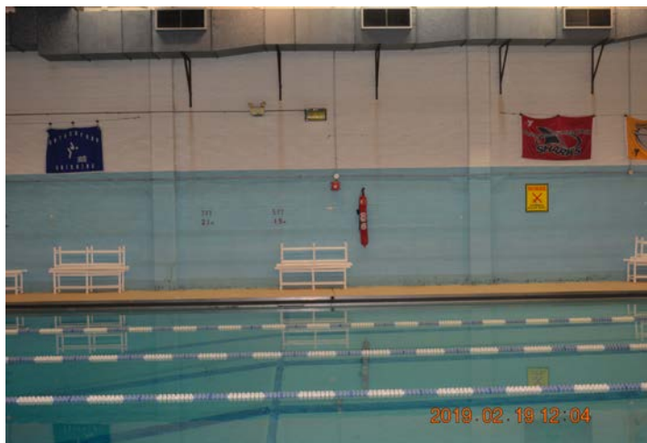
Photo 24: All metal items and fasteners suffer from corrosion as can be seen by the rust streaks below the duct support brackets on the opposite wall.
