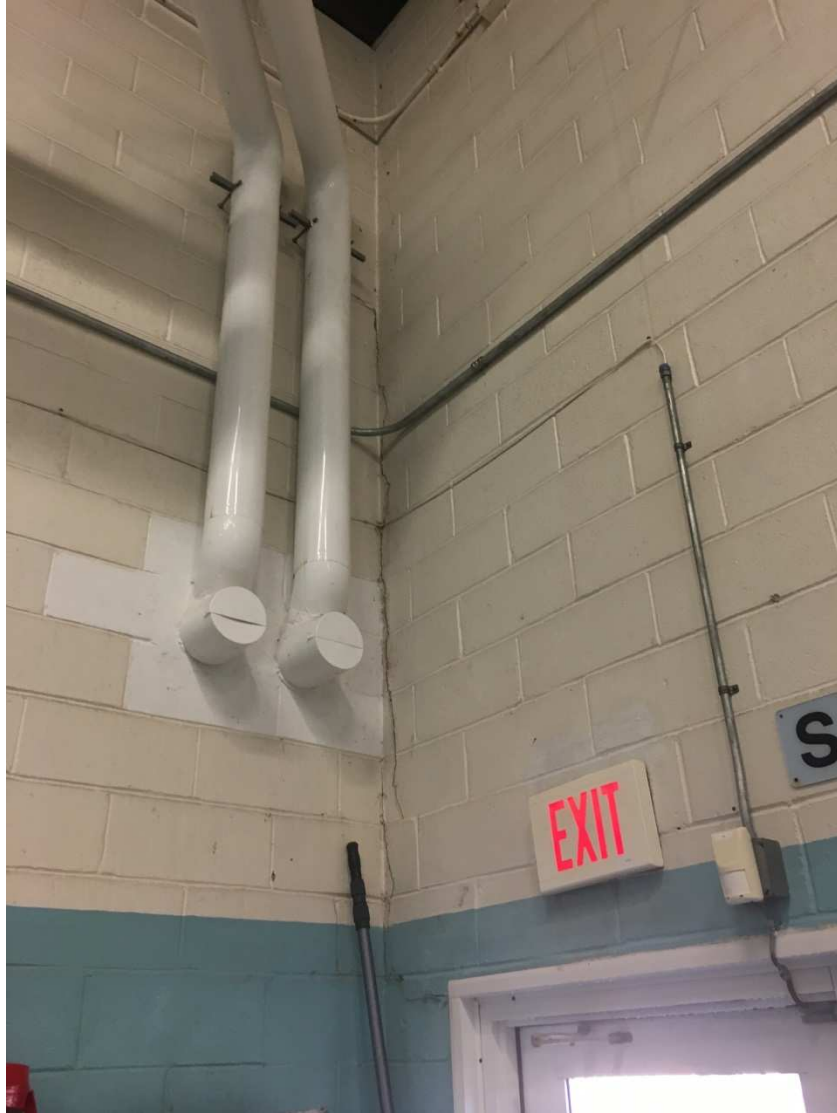
Photo 4 – Northwest corner, note crack in corner of walls.
